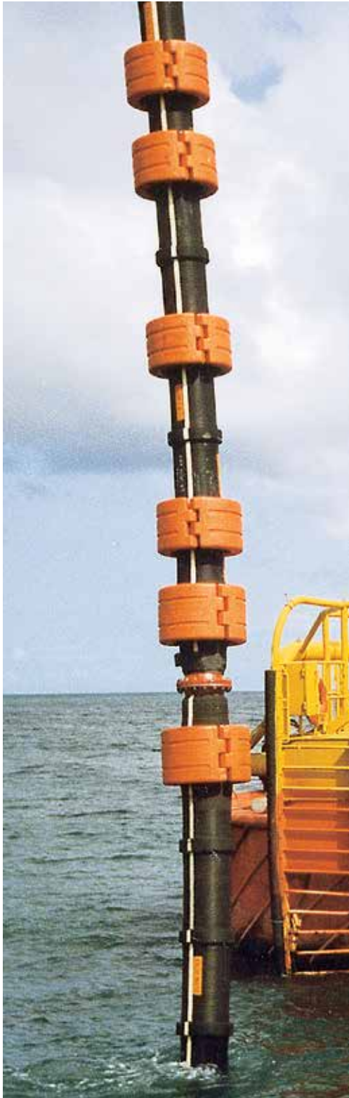
Trelleborg Marine Systems Submarine Hose Floats being deployed as part of a Single Point Mooring system.
