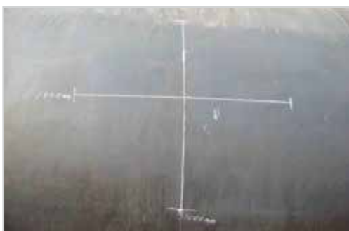
Circumferential and longitudinal mark
